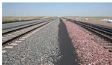
Note coal dust deposit in ballast drainage area Enlarge
