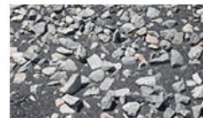
Coal dust in ballast section Enlarge
