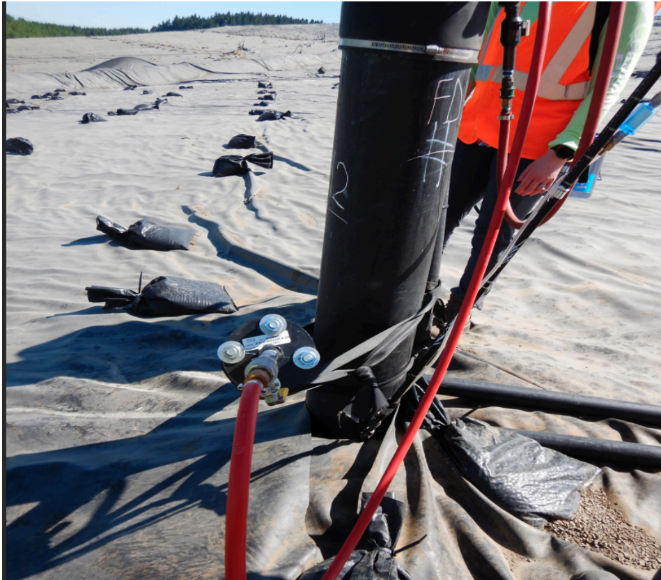
Example 1 - 4,000 ppm Methane Exceedance at gas collection piping/equipment
