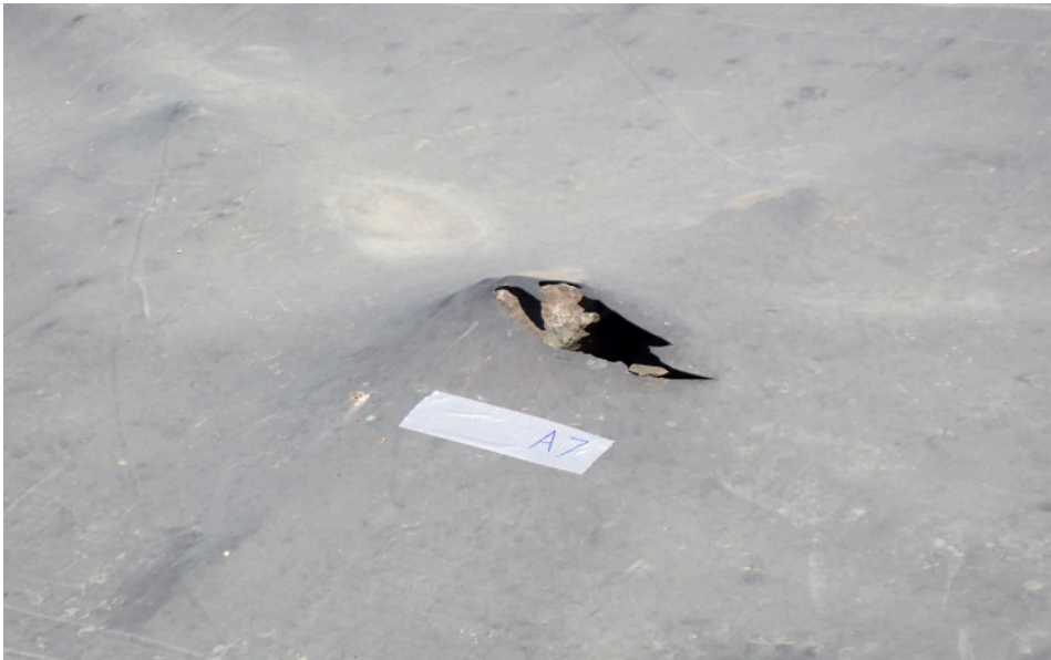
Example 2 - 20,000 ppm Methane Exceedance from small tear in the tarp
